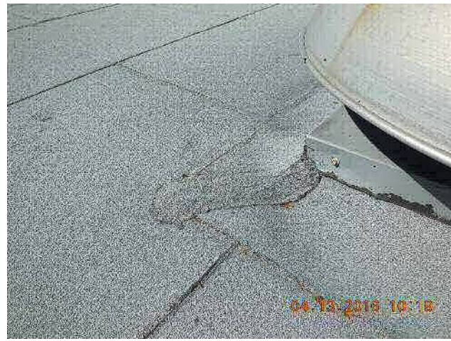
Visible Roof Discoloration at Vent
